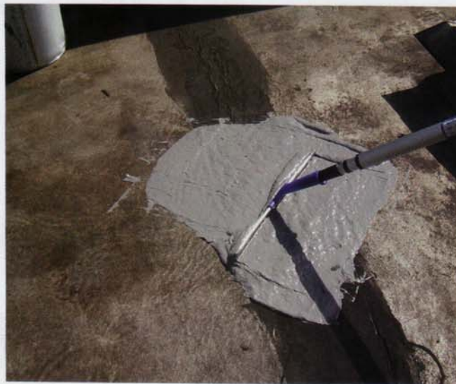
The ability to remain supple and capacity to move with the substrate is an essential attribute for a good roof covering
